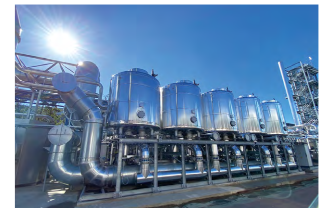
Nitto Belgium NV's energy-saving solvent recovery equipment
