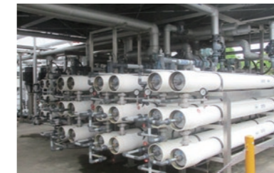
Water recycling facility at the Shiga Plant
