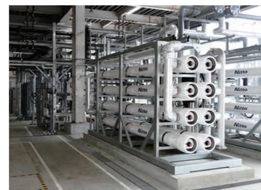
Water recycling facility at the Onomichi Plant
